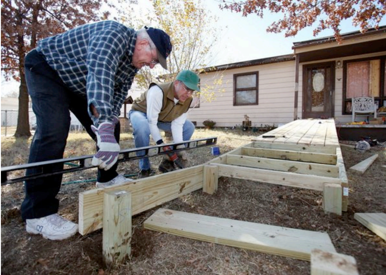
Wayne Tremble and Alan Sylvester level a ramp for a house. They are helping Dean Lesikar and Rebuilding Together Tulsa make a ramp for an elderly person earlier this week. STEPHEN PINGRY/Tulsa World
