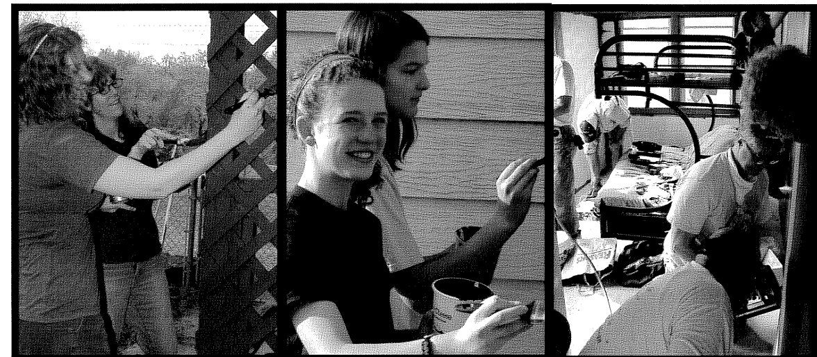
Left: Linda and Destiny Hrcir participated in order to give back. They were helped in a similar way several years ago. Center: Lauren Burkhalter and Hannah Walsh love to volunteer and help people. Right: Six volunteers repair water damage and turn a purple room white.
